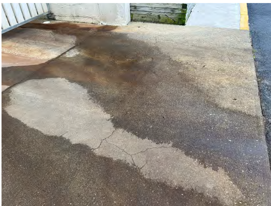
Photograph 26 – Cracks in trash enclosure concrete apron.
