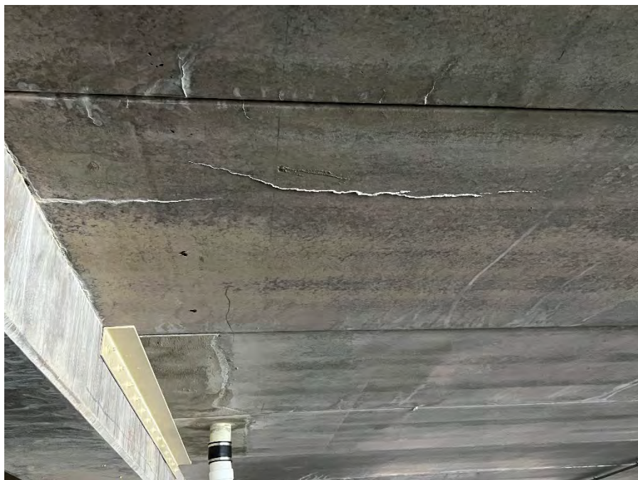
Photograph 15 – Calcium deposit in the soffit of the parking garage.
