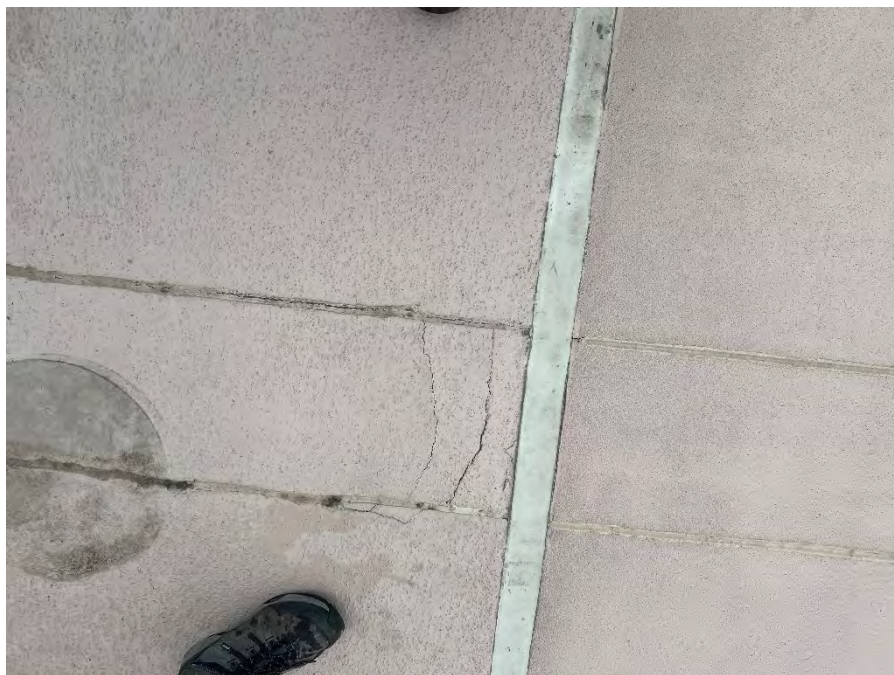
Photograph 13 – Cracks in terrace coating.
