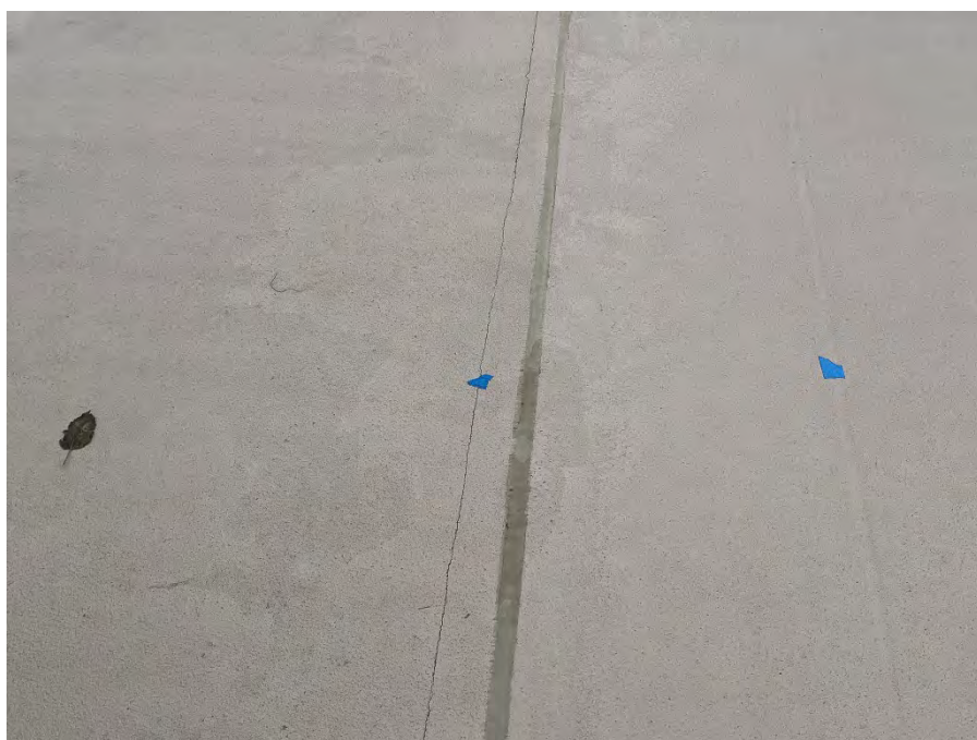
Photograph 12 – Crack in swimming pool deck coating.
