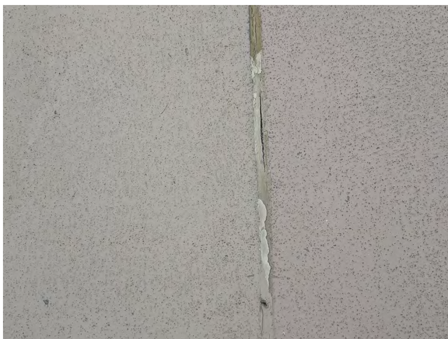
Photograph 14 – Debonded control joint sealant in terrace.
