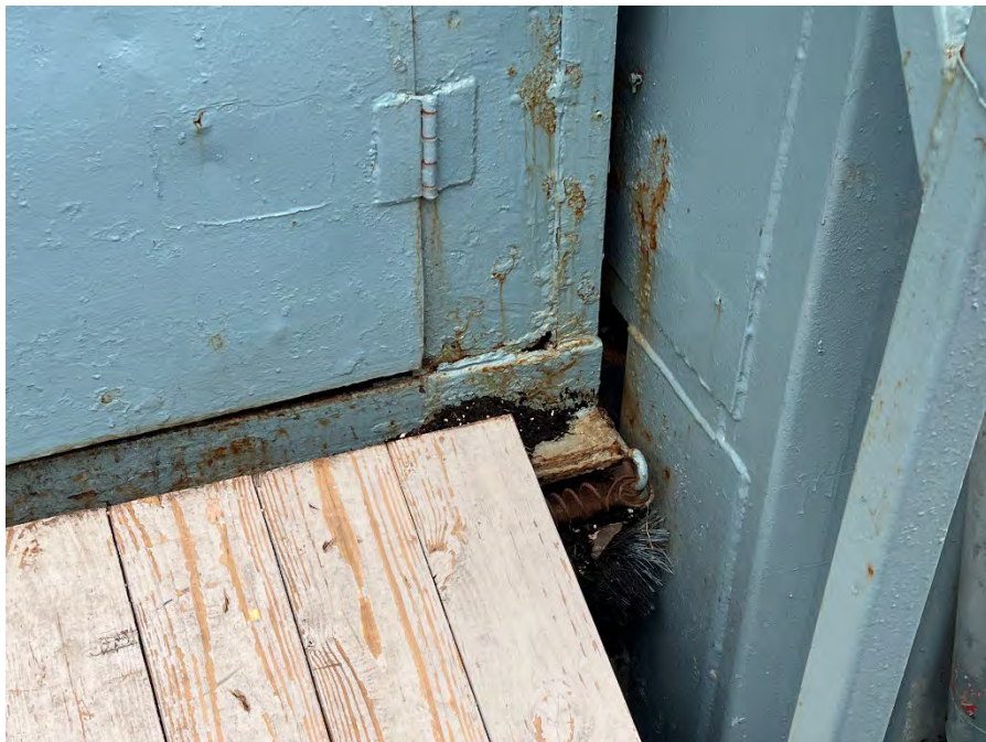
Photograph 19 – Corrosion on trash compactor.
