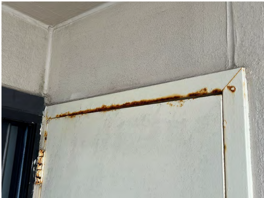
Photograph 7 – Corrosion on steel door
