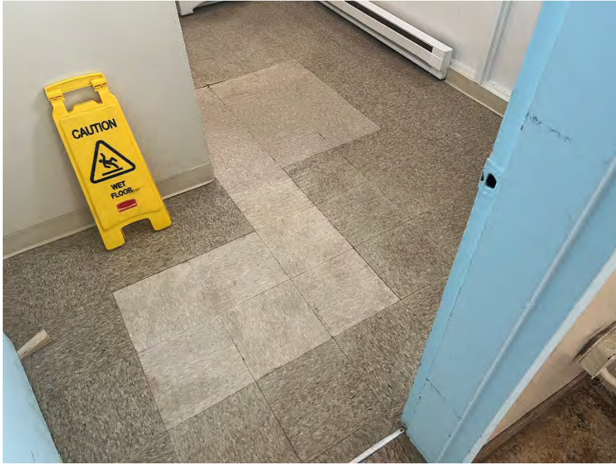
Photograph 21 – Mismatched tiles in the.
