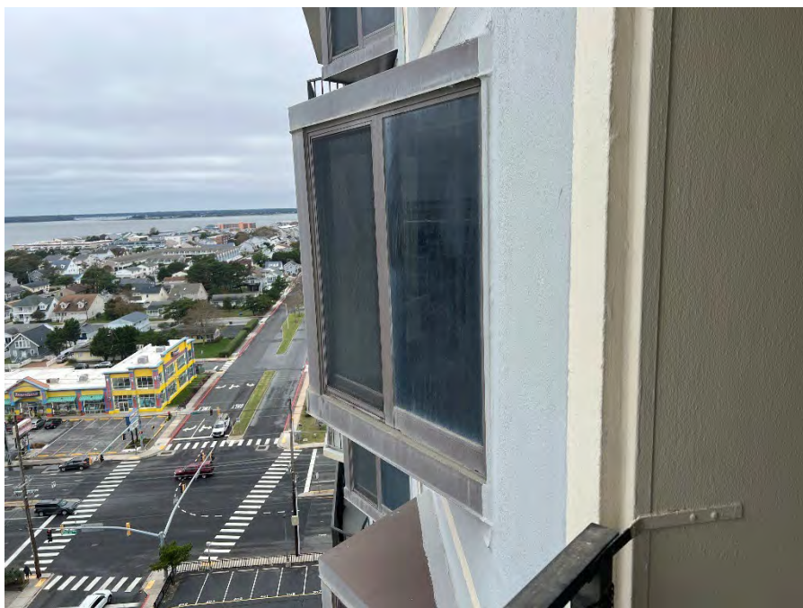
Photograph 6 – Faded color-coat on window.
