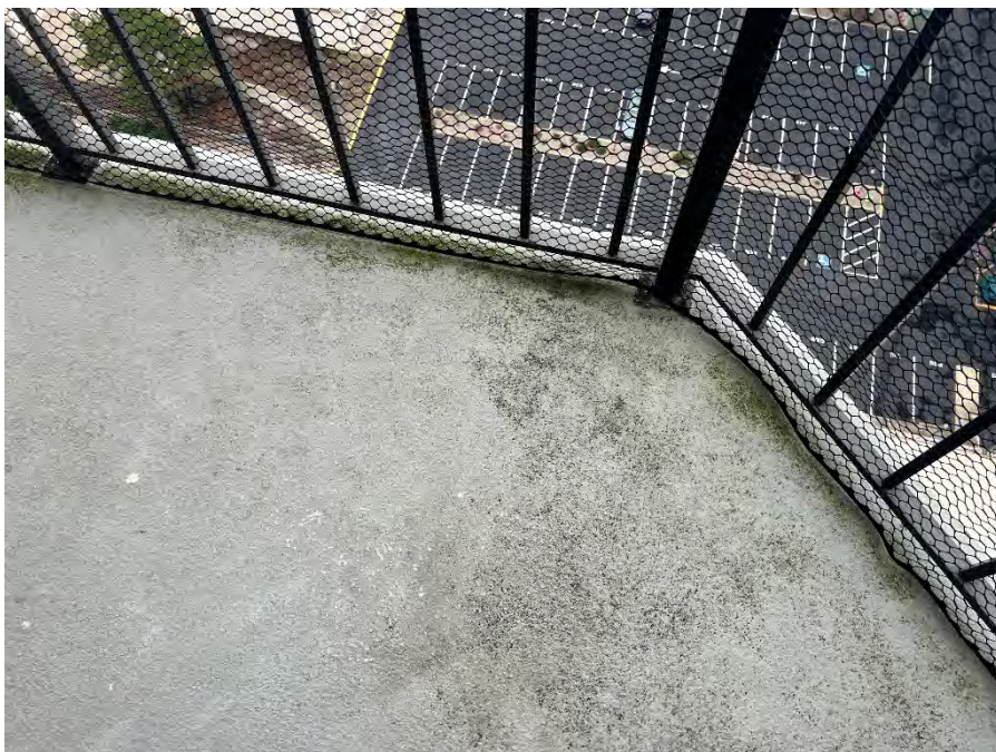
Photograph 9 – Staining on balcony.
