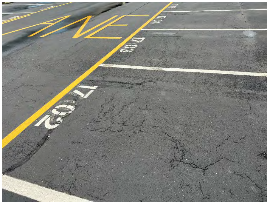
Photograph 23 – Interconnected cracks in asphalt pavement.
