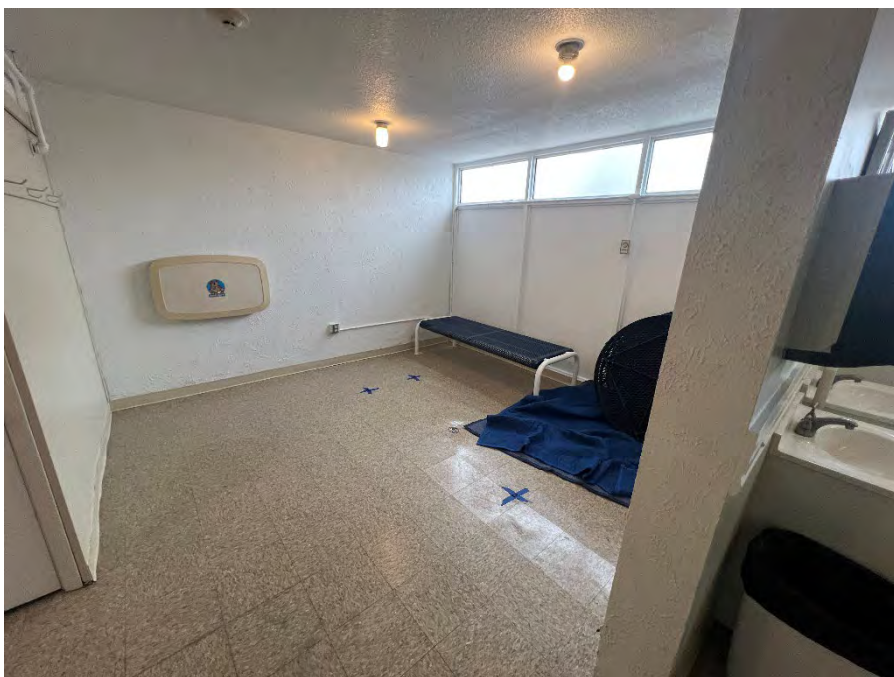
Photograph 20 – Debonded tile in the pool bathrooms.
