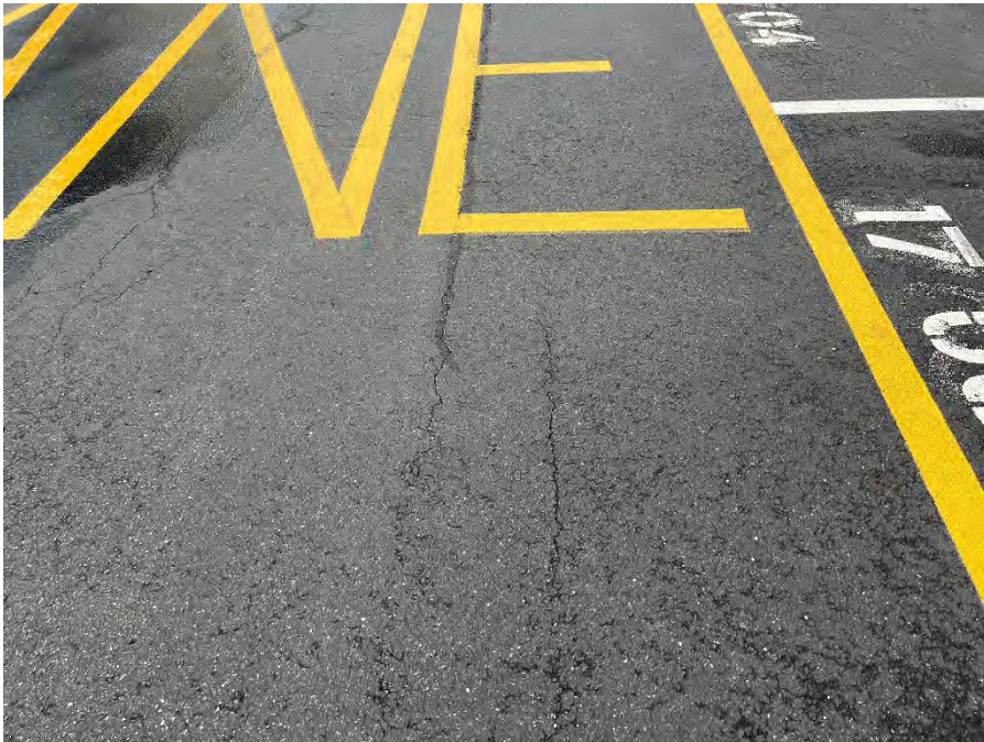
Photograph 22 – Simple cracks in asphalt pavement.
