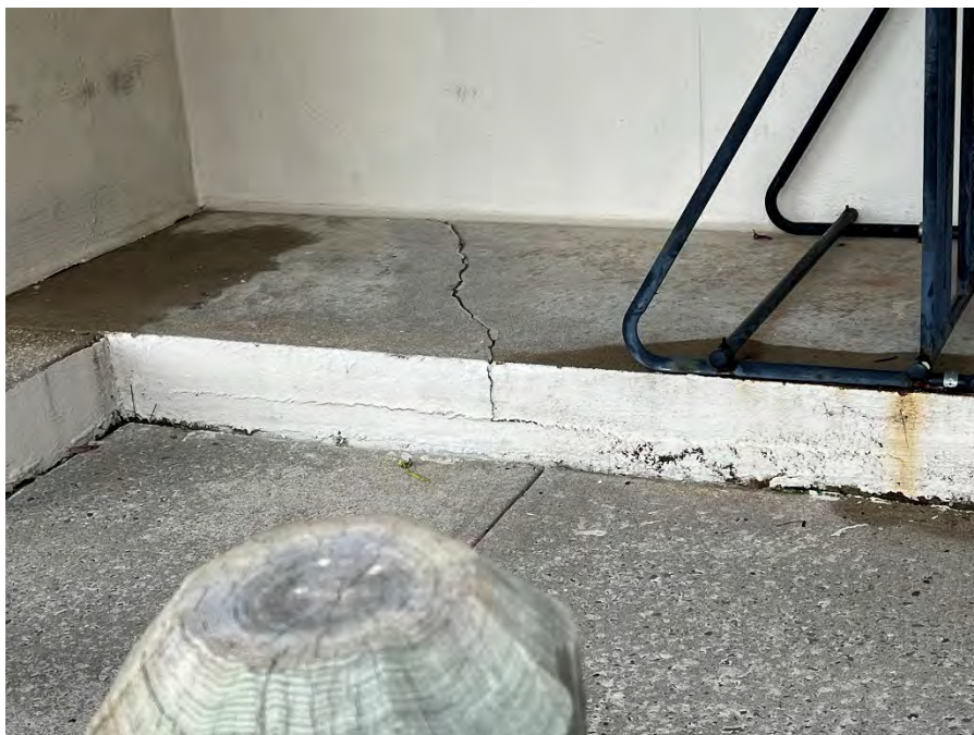
Photograph 25 – Crack in raised concrete walkway.
