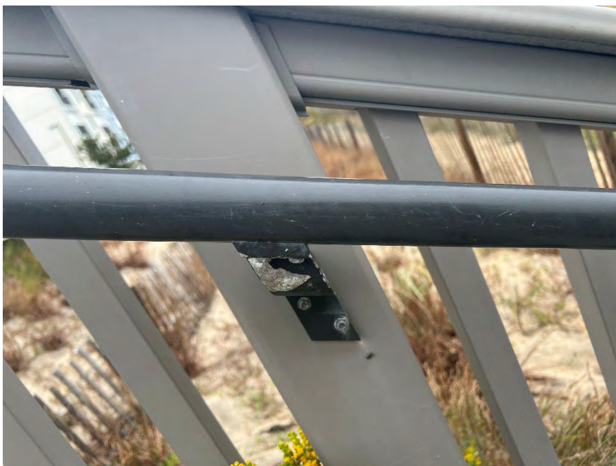
Photograph 18 – Debonded color-coat on stair assembly handrail leading to the beach.
