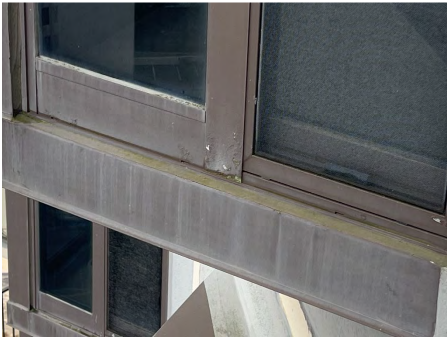
Photograph 5 – Debonded color-coat at base of window.
